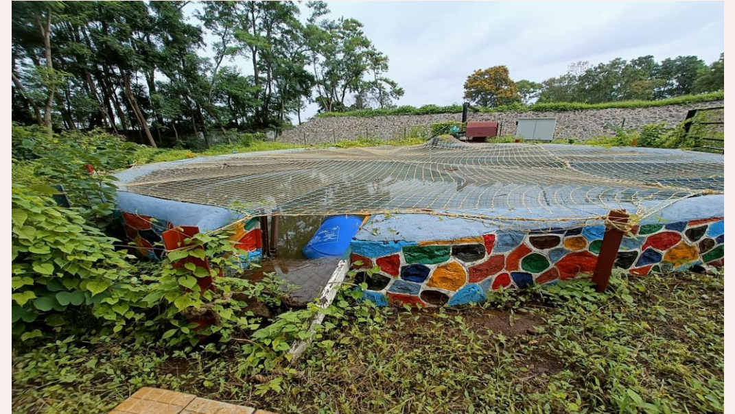
UG open Tank Capacity - 1 Million Litres
